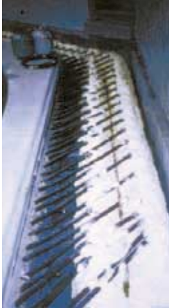
Insulating brine headers with foam prevents condensation on the surface, reducing corrosion, icing and frost heave.
