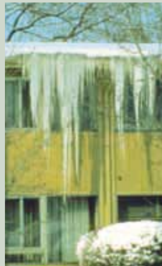
Ice damming can not only ruin a roof; icicles like these can be dangerous if they break off and fall.
