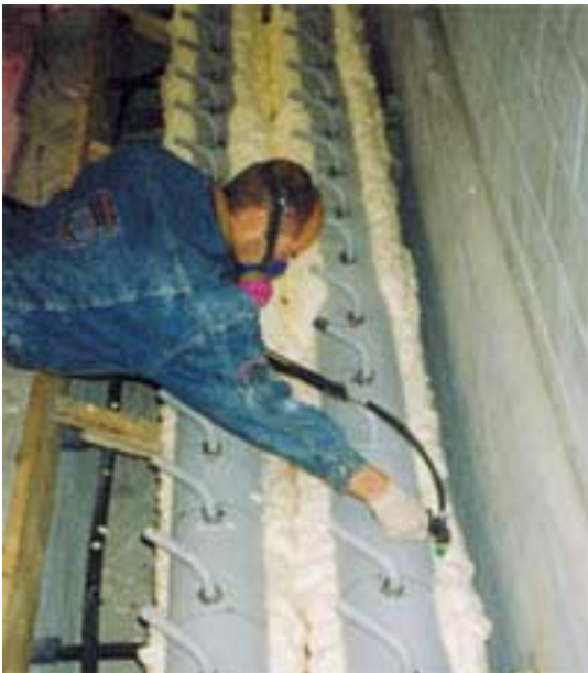
Canam uses a two-component polyurethane spray foam - the material of choice in this application.
