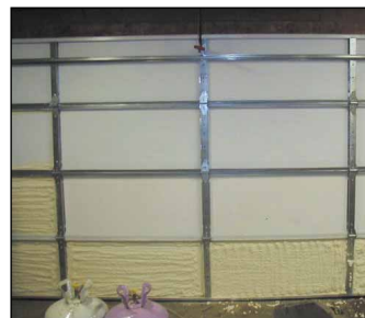
This garage door was coated with ZERODRAFT spray foam and is now an R-14 as well as being sealed. Vic reports this significantly changed the structure according to the owner.
