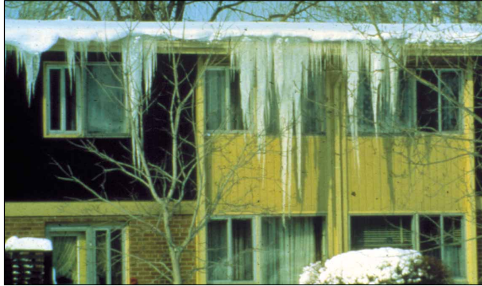
The Comfort Company prevents ice-damming problems like this with a comprehensive attic sealing package.
